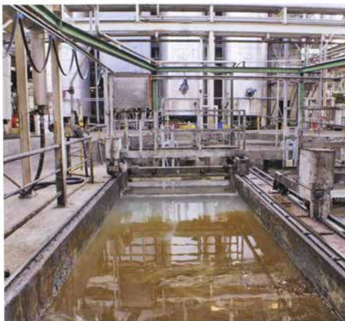
View of an oil and fat separator. The influent water is warm and contains a high load of mainly oils and fats.
