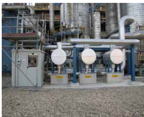
Figure 7: Analyser shelter with 3 each heat exchangers
