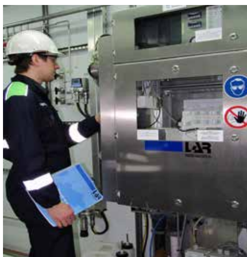
Figure 2: Inspection of a TOC-analyser in ATEX zone 1
